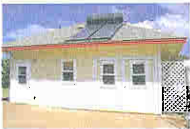
A solar water heating system at a West Maui residence uses energy from the sun to heat the family's water supply. "We never run out of hot water."
